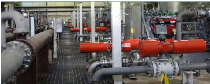
Inter-Stage Piping in Compressor Facility (Courtesy of Archer Daniels Midland Company)
