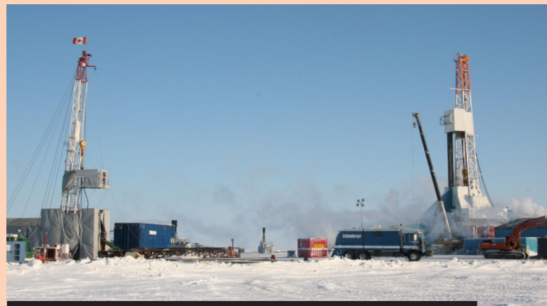
Figure TB-3.2: The Mallik Gas Hydrate Production Research Well, Mackenzie Delta, Northwest Territories, Canada. (Photo courtesy of the Geological Survey of Canada).
