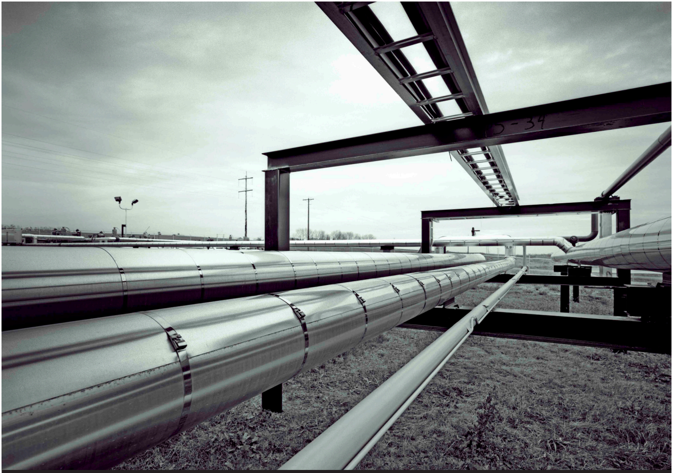
Figure 1.1: Natural gas infrastructure in northern Russia. (Courtesy of Lawrence Hislop, GRID-Arendal)
