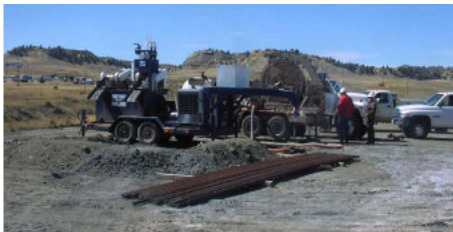
Microdrilling site at the Naval Petroleum Reserve No. 3. The Los Alamos drilling mud cleaning system and coiled tubing drilling rig are shown, from left to right.
