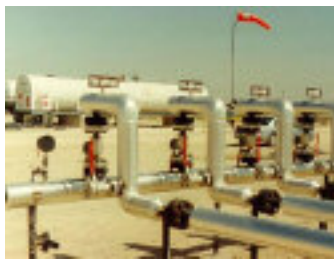
CO 2 gauging facilities at Lost Hills field.
