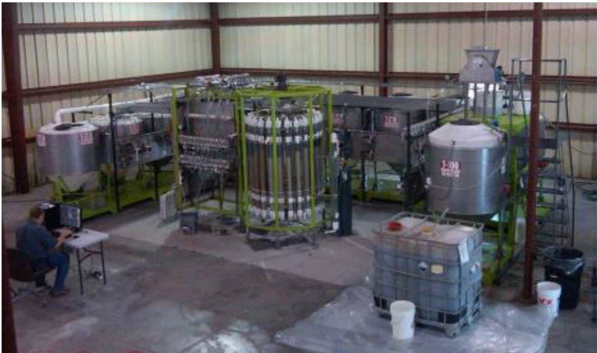
Continuous ion exchange pilot system.
