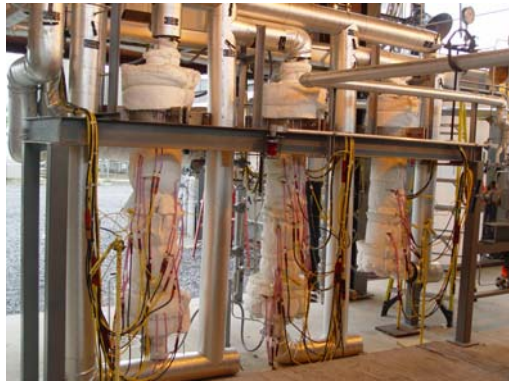
Figure 10. Small Reactors in Syngas Cleanup Facility.
