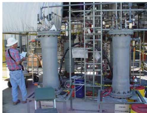
Figure 11. Solution Scrubbers in Syngas Cleanup Facility.
