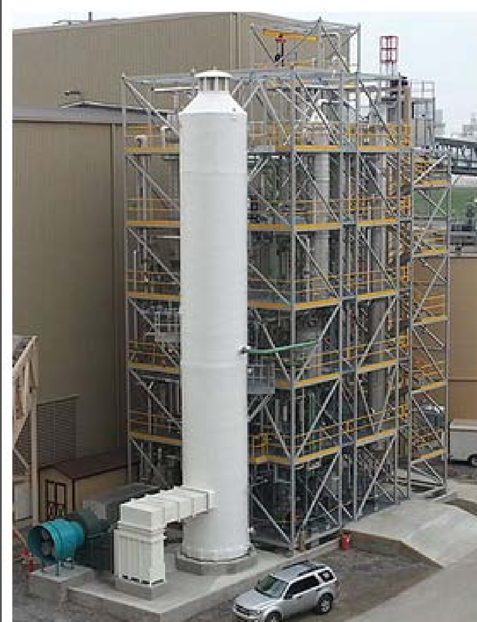
The 0.7 MWe slipstream testing facility
