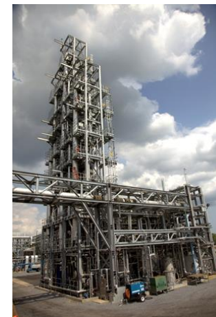
NCCC Infrastructure for 0.5 MW Pilot
