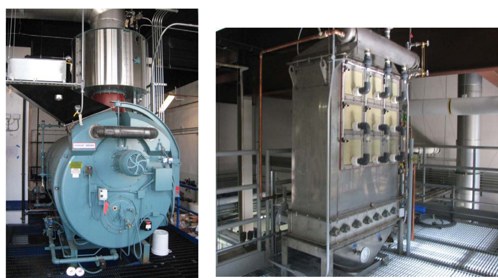
TMC Field Demo for Industrial Steam Boilers
