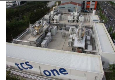
11.2 MW plant - largest fuel cell park in the world
