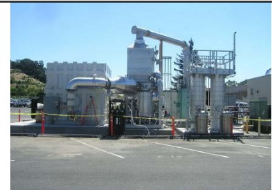
1.4 MW plant at a municipal building
