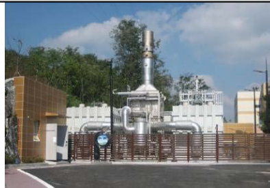
2.4 MW plant owned by an Independent power producer
