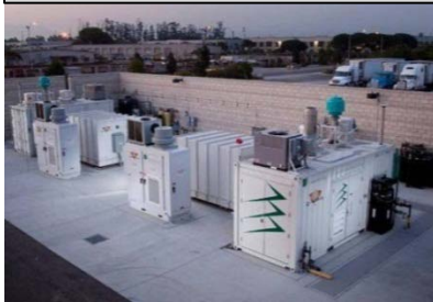
600 kW plant at a food processor
