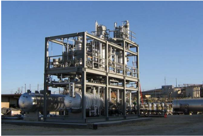
SulfaTreat DO (1.3 ton/day plant at Bakersfield, CA)
