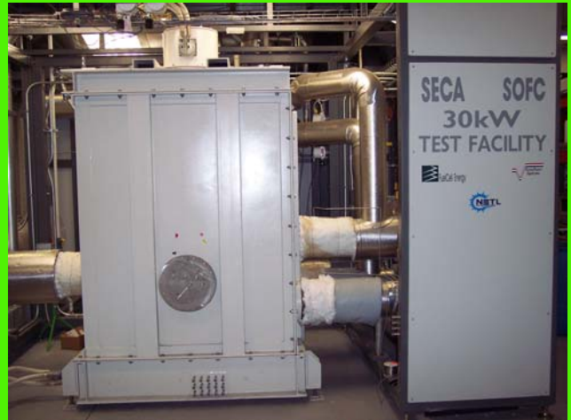
Test Facility for 15kW t SOFC/T Recuperator
