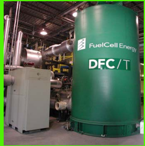
Test Facility for 150kW t DFC/T Recuperator
