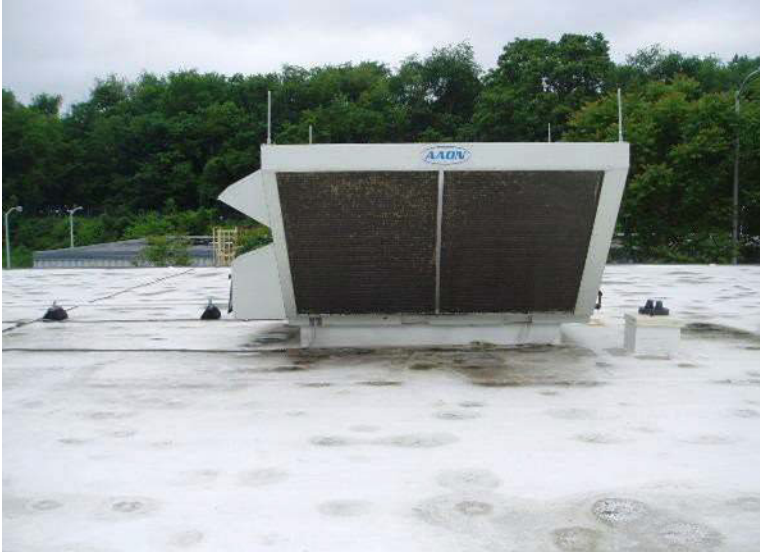
Photo 3.3.6.3: Pittsburgh Air Conditioner Condensate.
