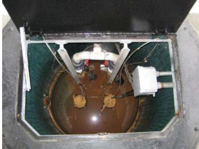
Photo 3.5.6.1a: Morgantown Parking Lot Oil-Water Separator.
