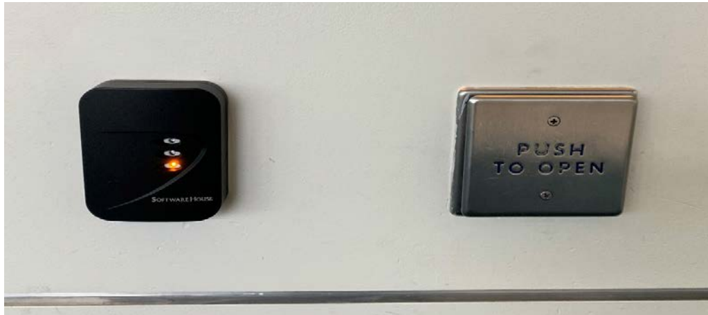
Photo 3.5.2.2a: Access Control Card Reader.
