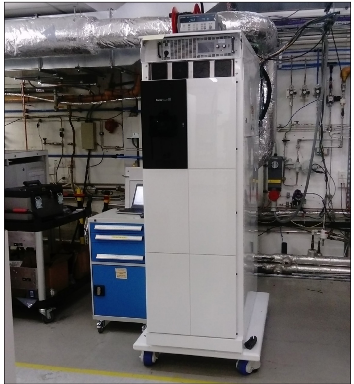
FIGURE 3. Cummins/Ceres Power 10 kWe SOFC System. Photo courtesy of Cummins/Ceres Power
