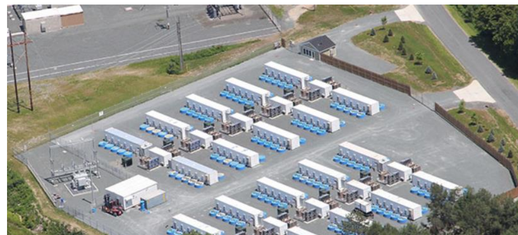
20 MW Flywheel Plant for NYISO
