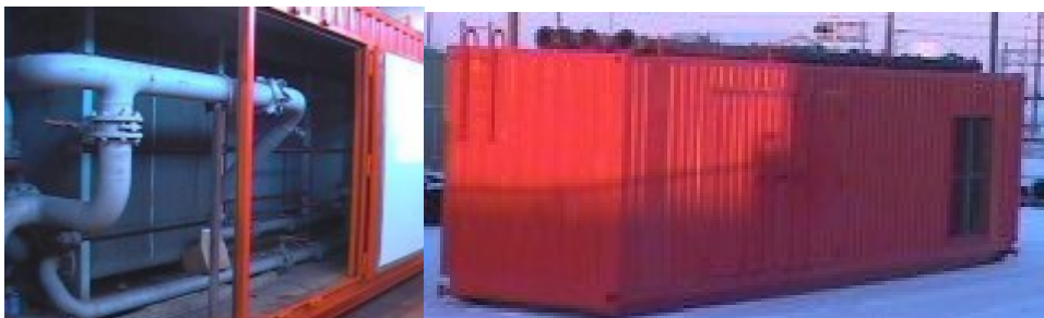
Figure 5: Photographs of commercially available mud cooler unit.
