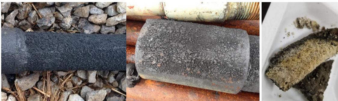
Figure 5. Calcium carbonate was detected on the downhole tubing (observed as the bumpy coating on the tubing (left and middle). The material was collected and sent to Montana State University for analysis (right).
