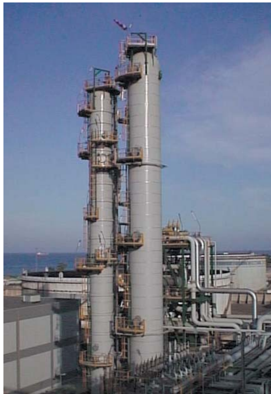
Fig. 43. Selexol unit at Sarlux plant, Sardinia.
