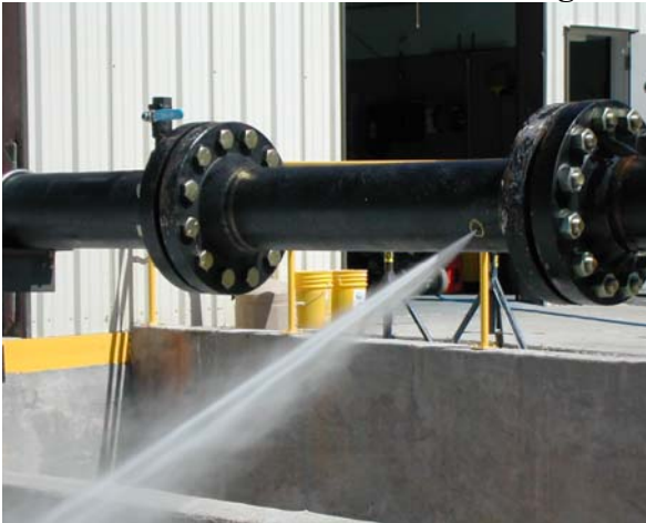
Photo 6: Internal Corrosion Leak Rate Testing
