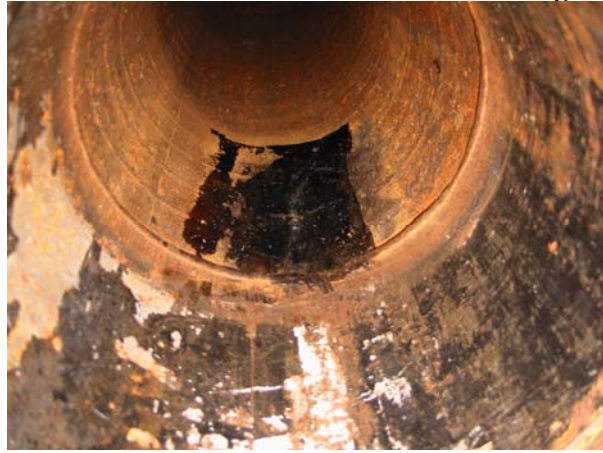
Photo 21: Internal Corrosion Defect with Flex-Plug
