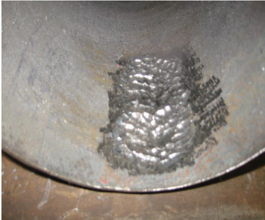
Photo 20: Internal Corrosion Defect - Bare
