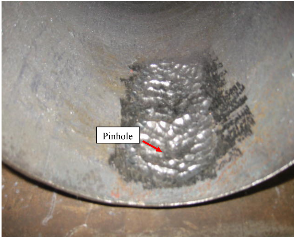
Photo 3: Internal Corrosion Defect
