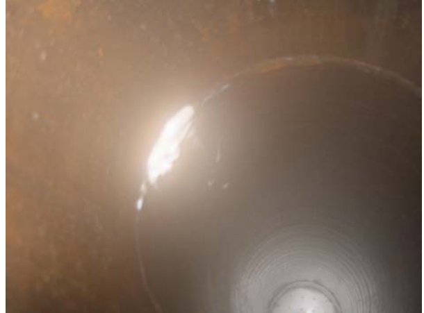
Photo 16: Soft Sealant Lump
