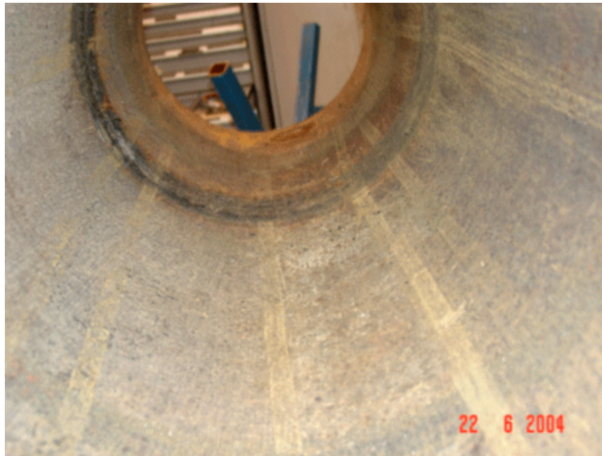
Figure 9. Cast-Iron Pipe ID after Cleaning
