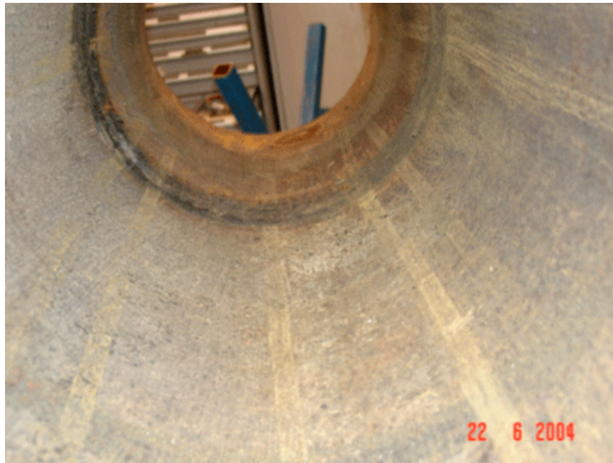
Figure 9. Cast-Iron Pipe ID after Cleaning
