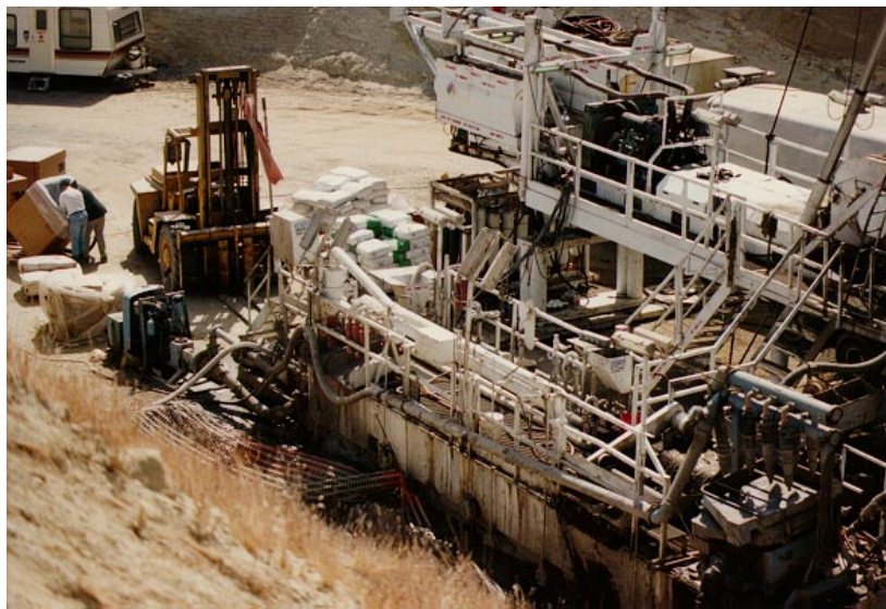
Fig. 20. Golden State Drilling Rig Mud System
