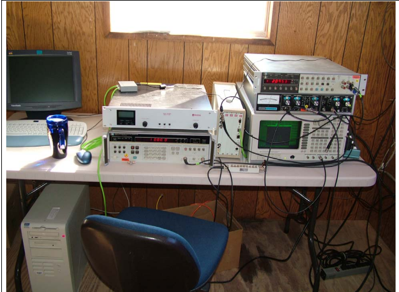
Figure 16. Photograph of test electronic in the vault
