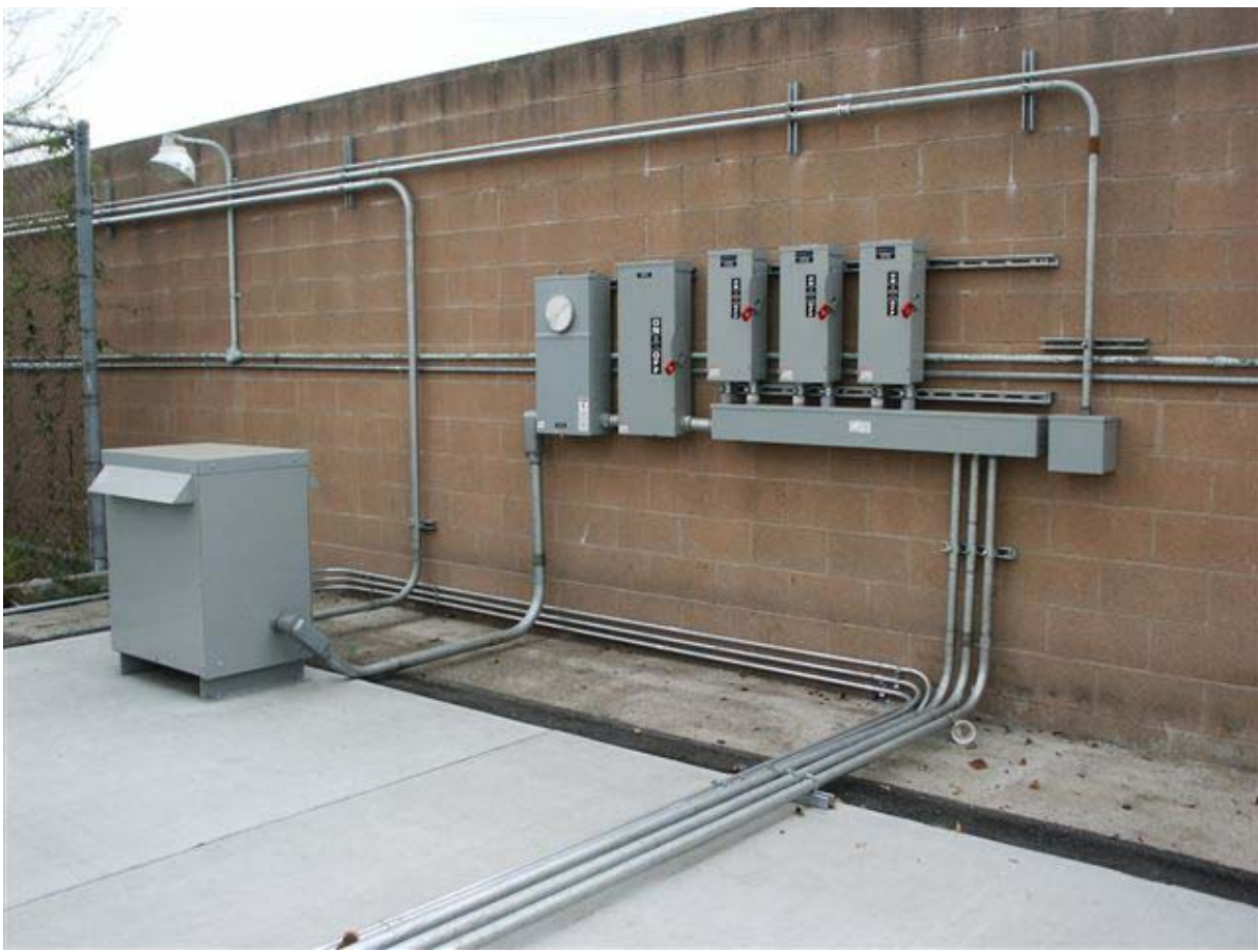
Electrical interconnection with Transformer
