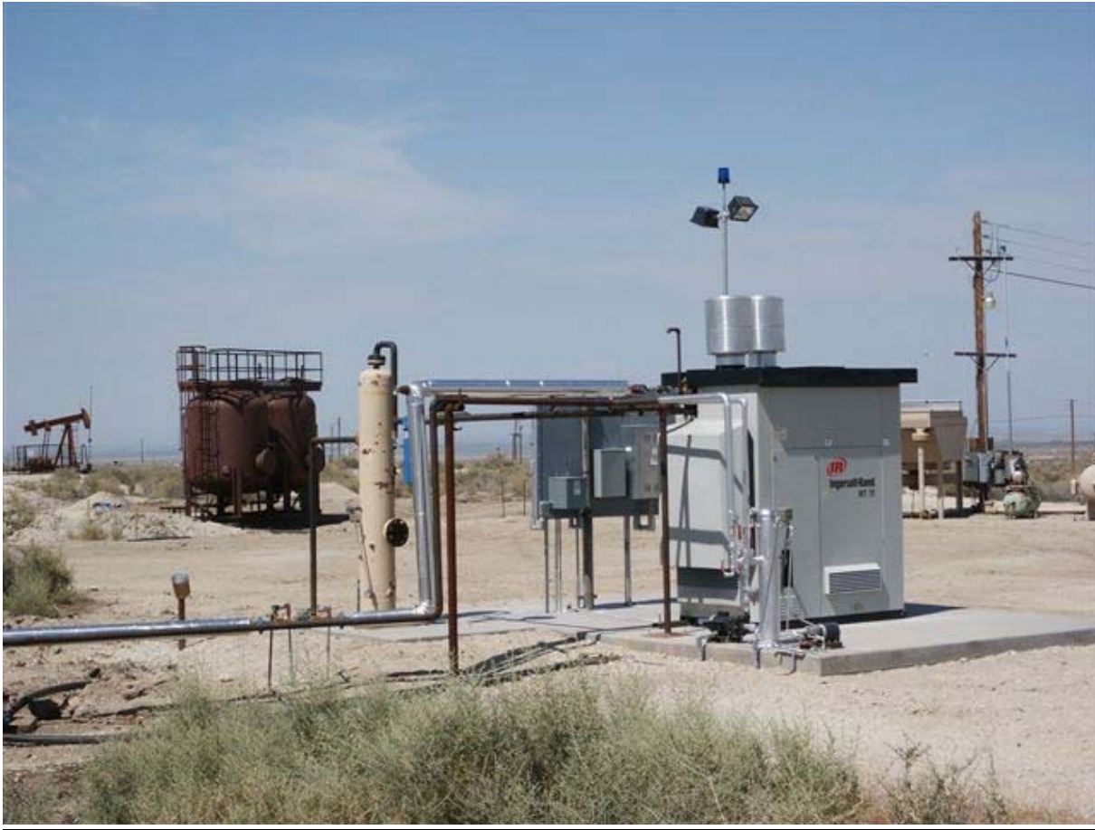
IR 70 with CHP Heat Loop
