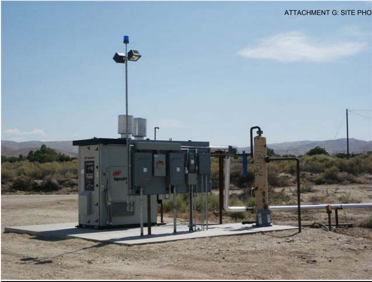
IR 70 with Vertical Free Water Separator and CHP Heat Loop
