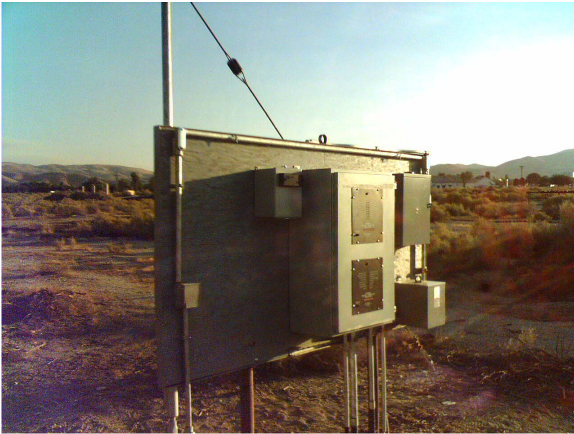
Double Redundant Beckwith Controller
