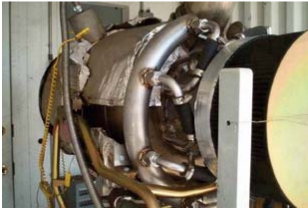
A 30 kW flex microturbine is now generating electricity on a California oilfield by burning ultra-low-BTU gas.
