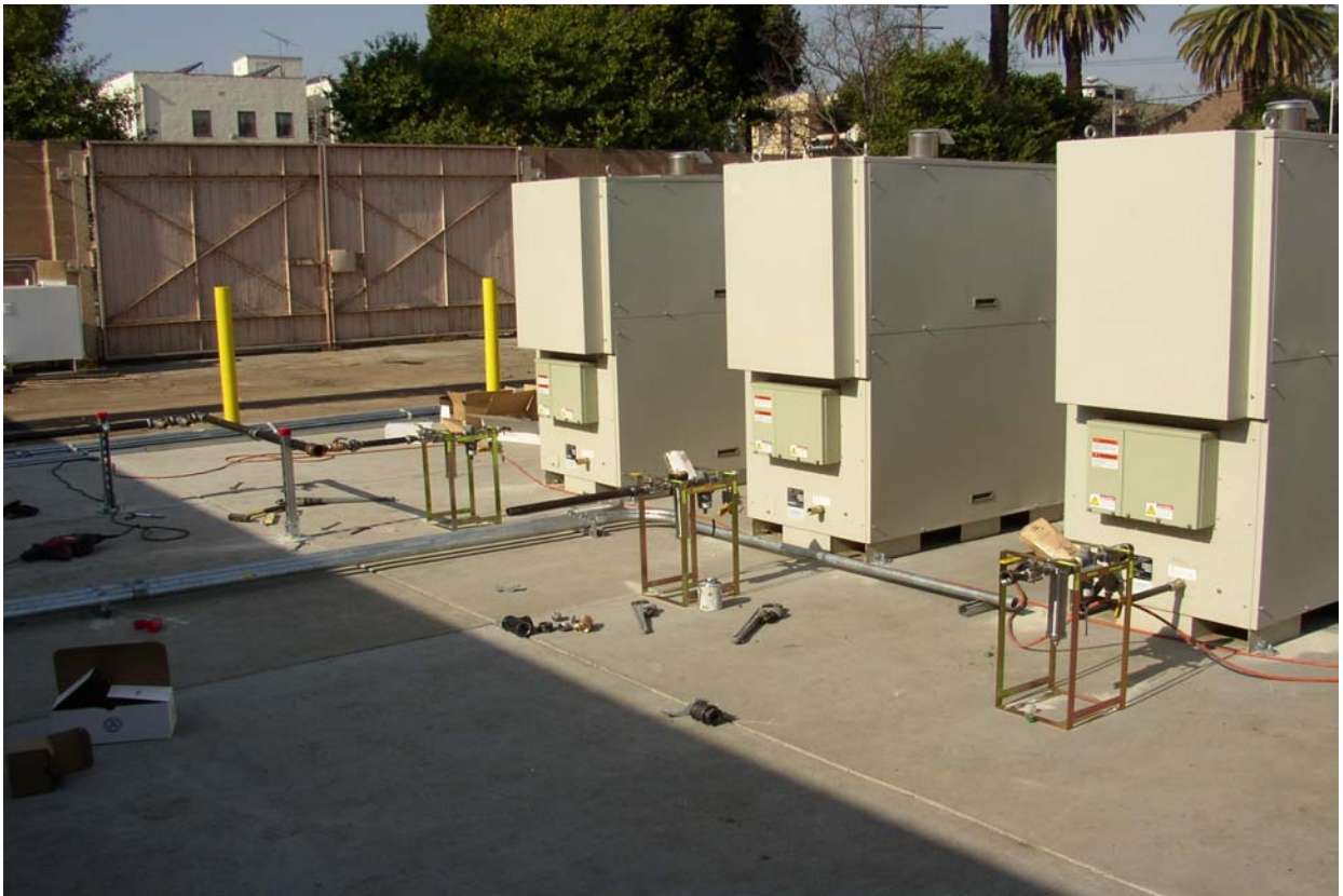
Rear Plumbing of C30 Units
