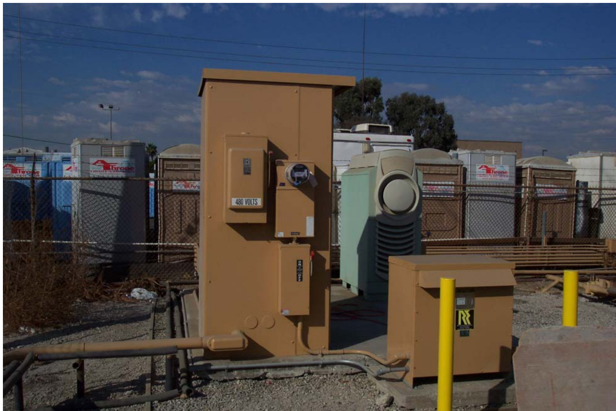
Capstone C30 Turbine with Electrical Interconnection and Transformer 57
