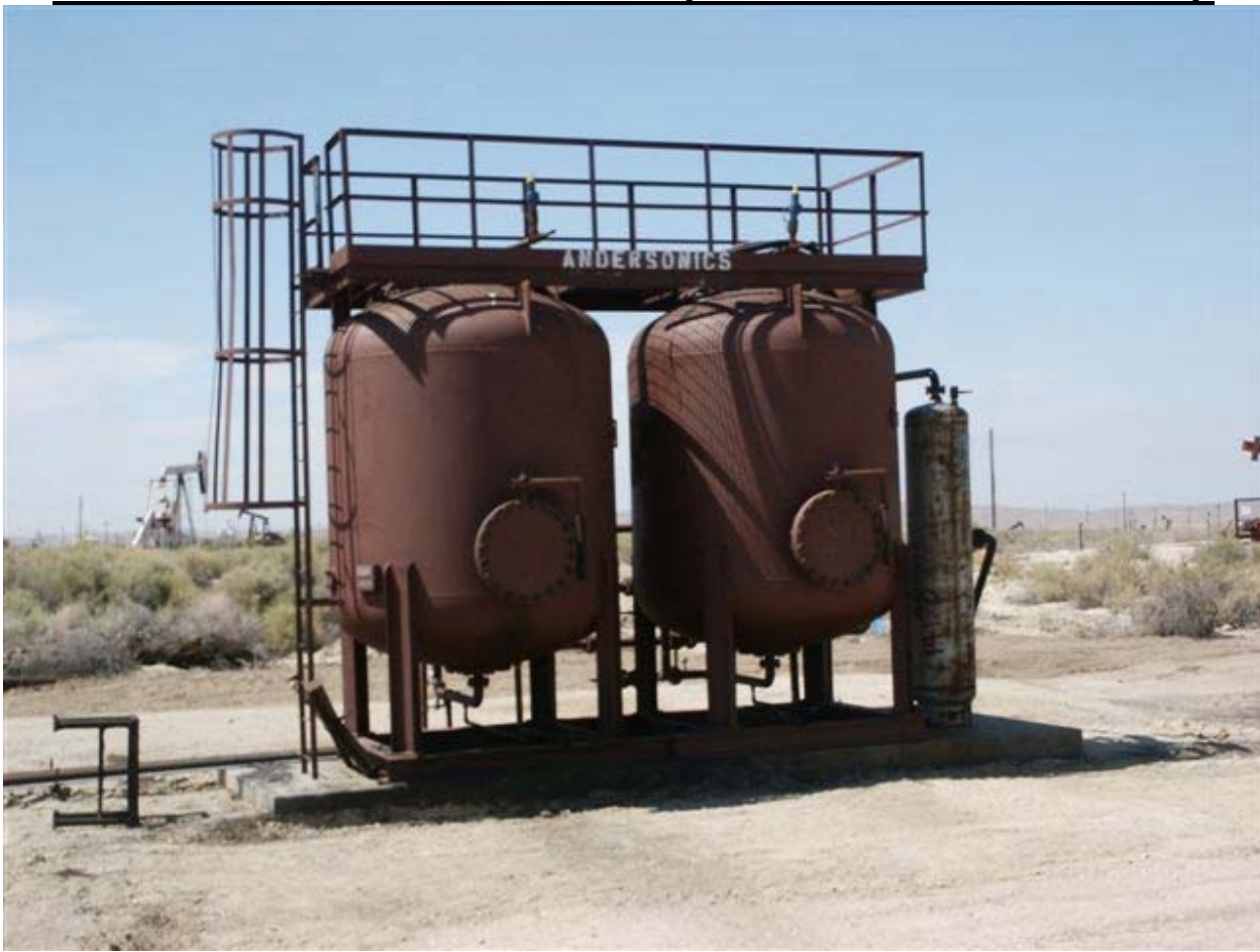
Sulfa-Treat Vessels with Lead/Lag Piping for Continuous Use
