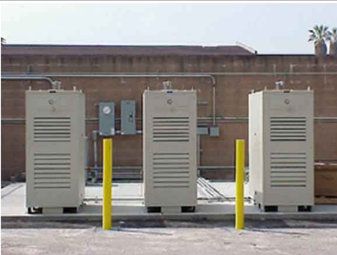
Three Capstone C30 Microturbines installed
