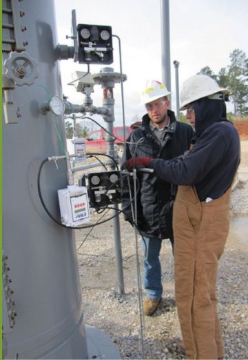
Researchers measuring the gas leakage rate on a pneumatic controller, a source of vented emissions, that relies on pressurized natural gas to control the opening and closing of a valve on a separator.
