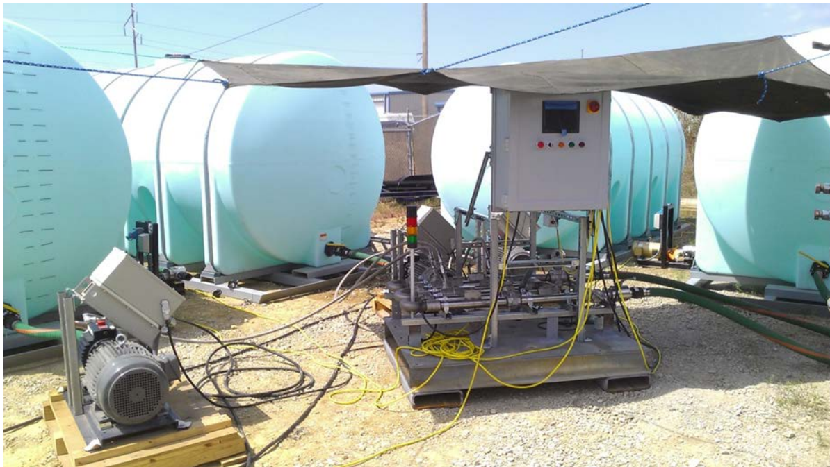
Figure 15. Full SPI Slip-Stream equipment Setup in Impact's Yard during Testing
