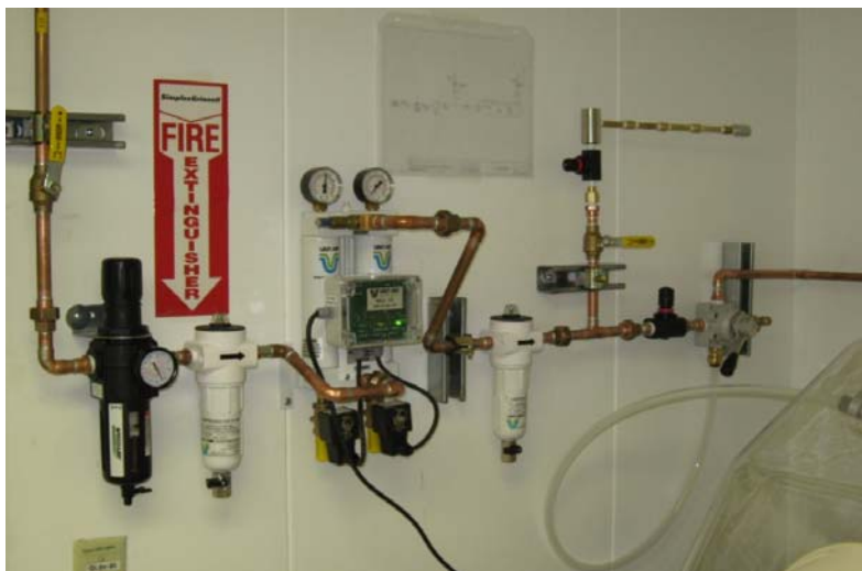
Figure 2. Picture of air supply system with regenerative desiccant air drier system
