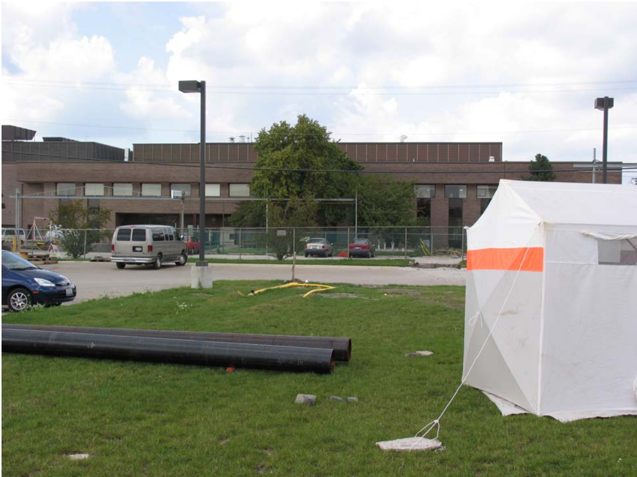
Figure 4: RFEC testing on 12" pipe samples.
