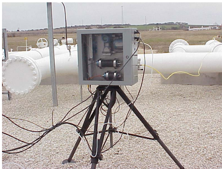
Figure 6-25. Front view of the energy meter module installed at the New Braunfels, Texas field site.
