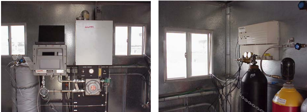
Figure 6-26. Field site enclosure for the on-site gas chromatograph (left) and the energy meter Bristol Babcock flow computer (right).
