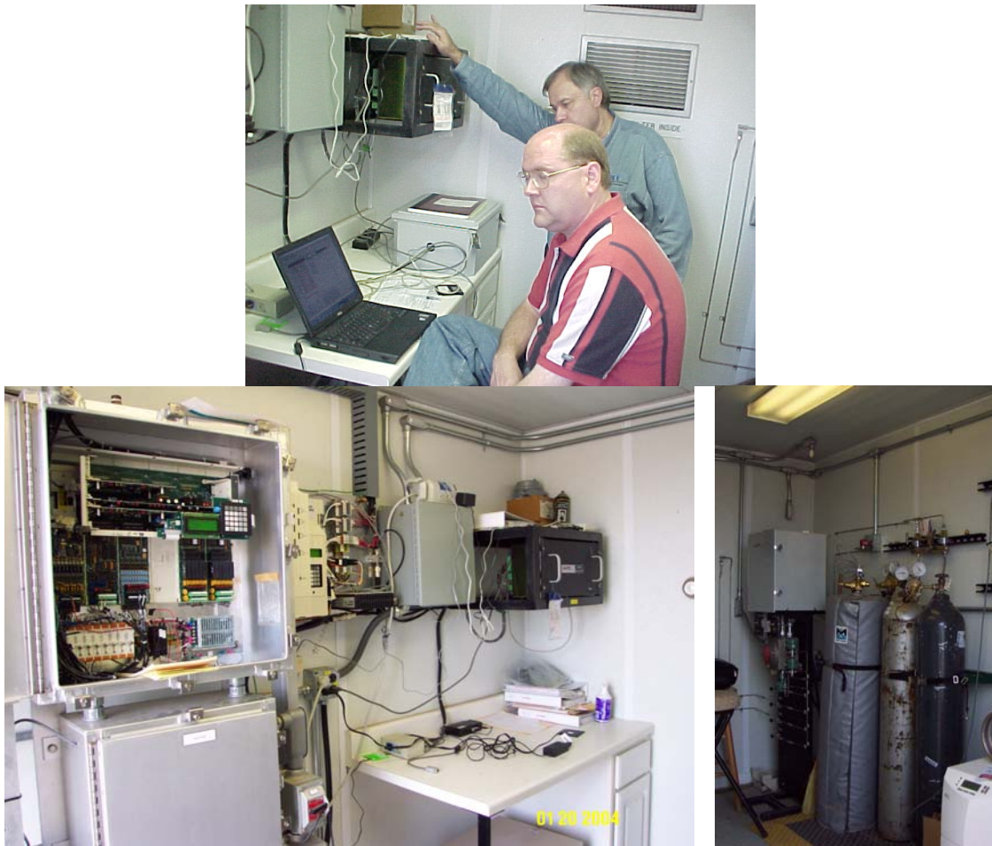
Figure 6-33. Installation of the RGC data logger at the El Paso field site. Top : RGC data logger (on the workbench) implementing the algorithm. Bottom left : Flow computer and data connections providing sound speed, temperature, and pressure data. Bottom right : Chromatograph providing diluent data.
