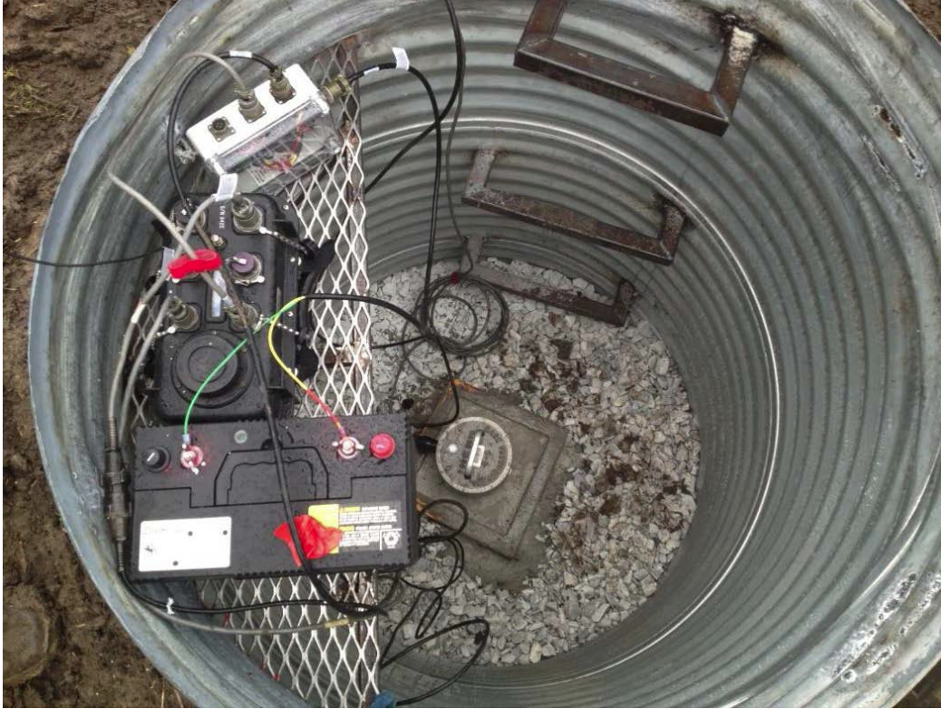
Figure 1.2 Photograph of seismometer vault installation at Wellington field showing Sercel L-22 seismometer, Data Acquisition System (DAS) Reftek RT-130, and power supply. (Peterie, 2014, Personal Communication).
