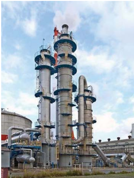
Amine Scrubbing Technology 330 ton CO 2 /day
