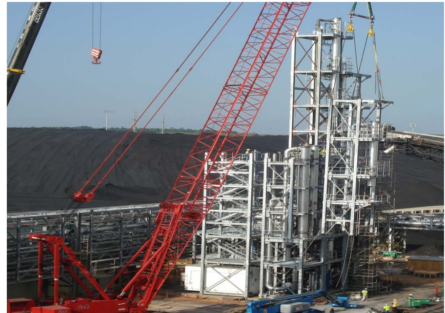
Post-combustion CO2 capture facility
