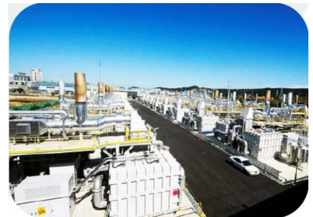
Hwaseong, South Korea 59MW Fuel Cell System
