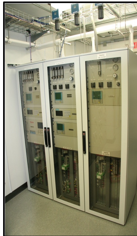
Analyzer and sampling panels
