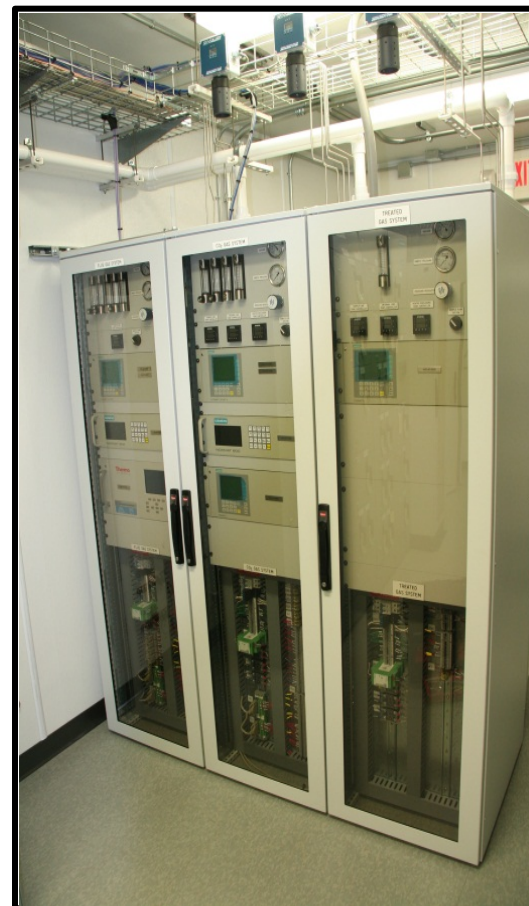
Analyzer and sampling panels
