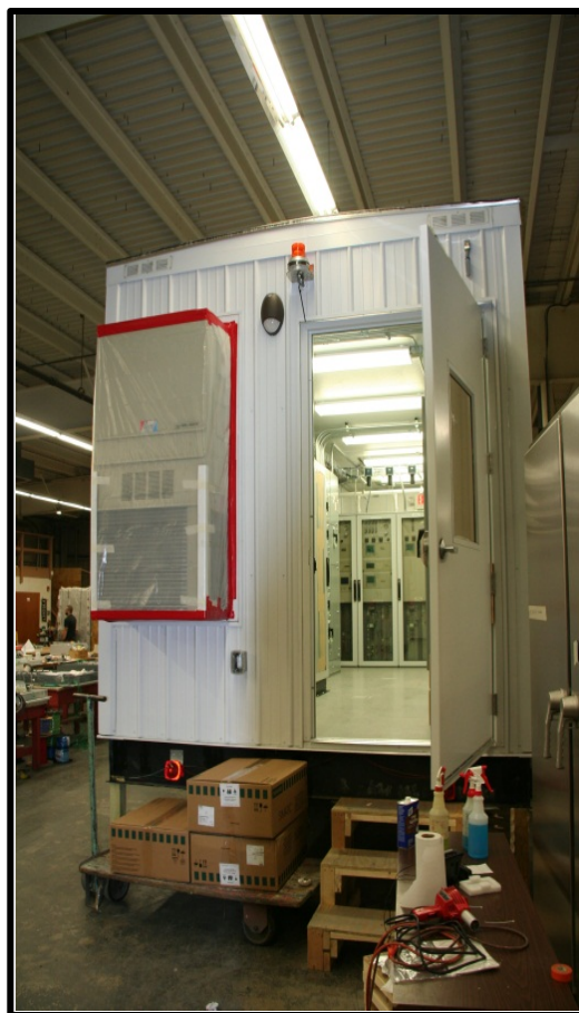
Analyzer and controls container
