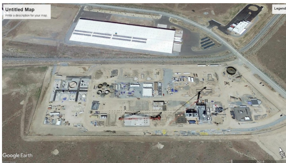
Exhibit B-8. Fulcrum Bioenergy 800 BPD Sierra BioFuels Plant (MSW to liquids) in Storey County, Nevada, United States
