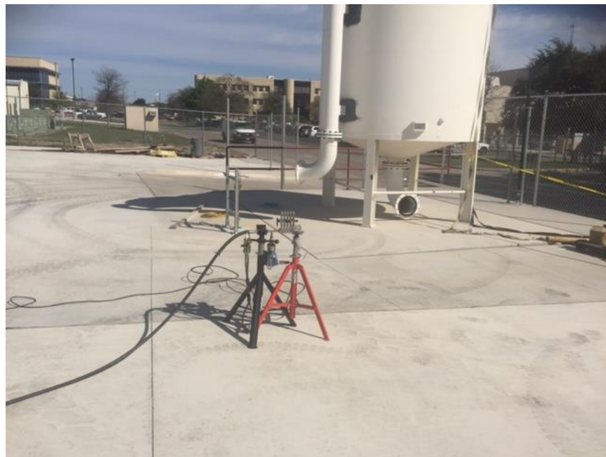
Figure 3: Controlled Methane Release Valves
