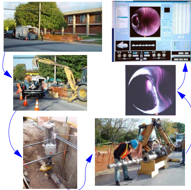
Figure XVIII : Explorer-I live deployment in a medium-pressure steel main
