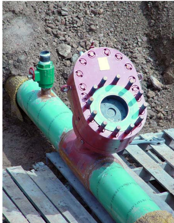
Figure LXXII :Angled live-launch launcher- and antenna-fittings and gate-valve installed on a live buried pipeline
