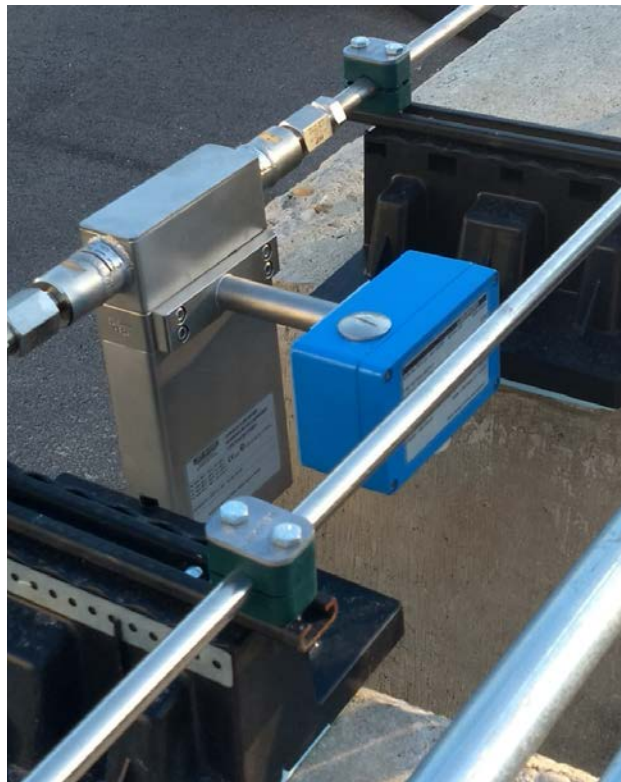
Figure 2-3 Rheonik RHM04L Coriolis Flow Meter Installed in Rheometer Section
