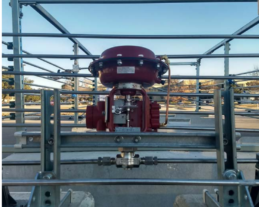
Figure 2-4 Research Control Valve HP-1711 Control Valve Installed in Rheometer Section
