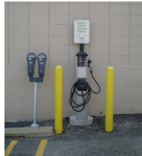
Figure 3. Example of AC Level 2 Public Charging Station Installed by MGE
