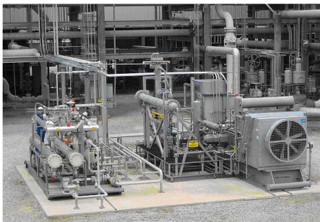
Picture of an MTR membrane test skid similar to one that will be built for a \text{CO}_2 capture demonstration unit to be installed at APS' Cholla, AZ, coal-fired power plant.
